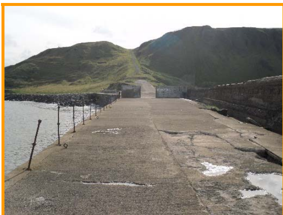
Looking landward along the jetty, showing open gates in background (Asset Ref No. 1221D901D0201C02)
