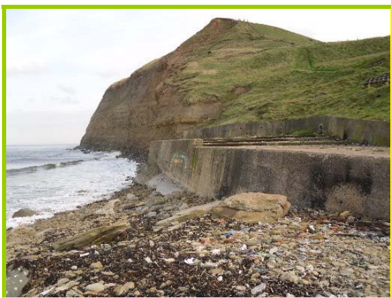
Beach ridge with concrete wall beyond (Asset Ref Nos. 1221D901D0202C04 and 1221D901D0202C03)
