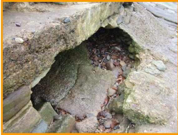
2008: Undercutting and excavation of concrete defences (Asset Ref No. 1221C901C0704C05)
