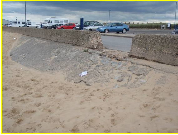
Gap in concrete wall and exposed revetment (Asset Ref No 12221C901C0601C01)
