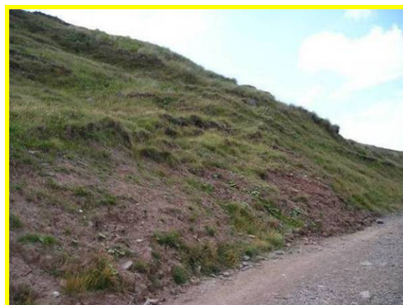
E56/1 recent activity at the cliff toe (Locally Active)
