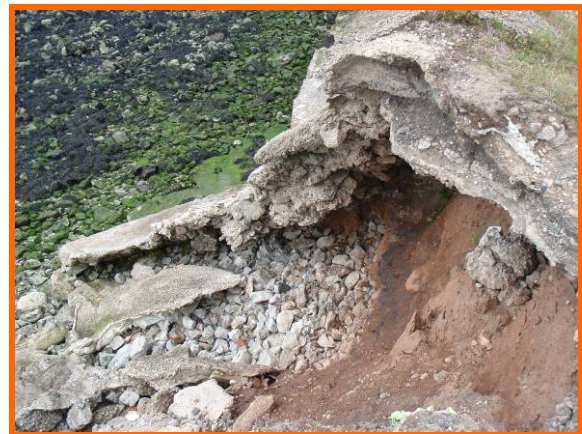
Undercutting of slag embankment on west side of structure (Asset Ref No 12221C901C0506C01)
