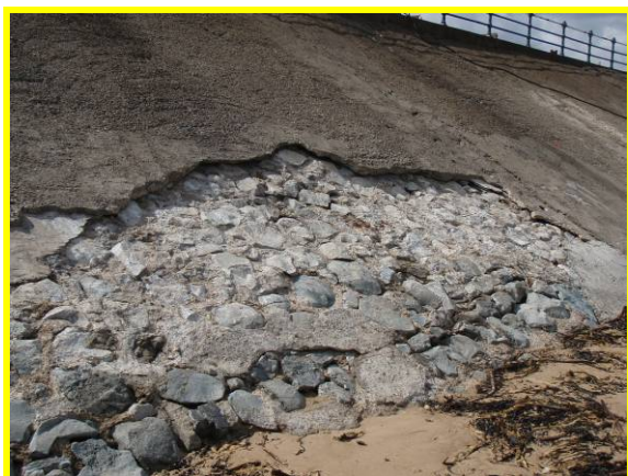
Loss of concrete render exposing grouted stone with minor voids (Asset Ref No 1221C901C0602C01)
