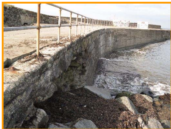
Looking seaward along the jetty, washout visible in foreground (Asset Ref No. 1221D901D0201C02)
