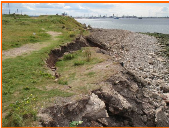
Extensive local slope failure on west side of structure (Asset Ref No 12221C901C0506C01)
