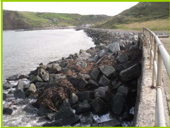
Tightly packed rock armour in good condition, from jetty to village (Asset Ref No. 1221D901D0202C01)
