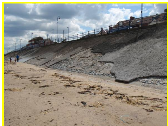
Loss of concrete render. Local infill repairs evident (Asset Ref No 1221C901C0602C01)
