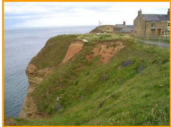
E59/1 and E60/1b cliff repairs in the till cap at Cowbar (Partly Active)
