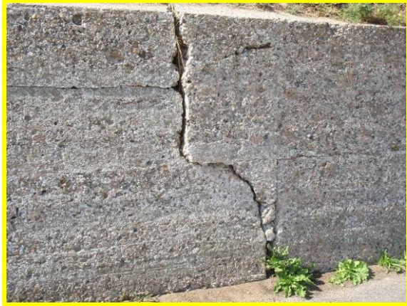
Crack in concrete wall below coastal slope (Asset Ref No 12221C901C0702C03)
