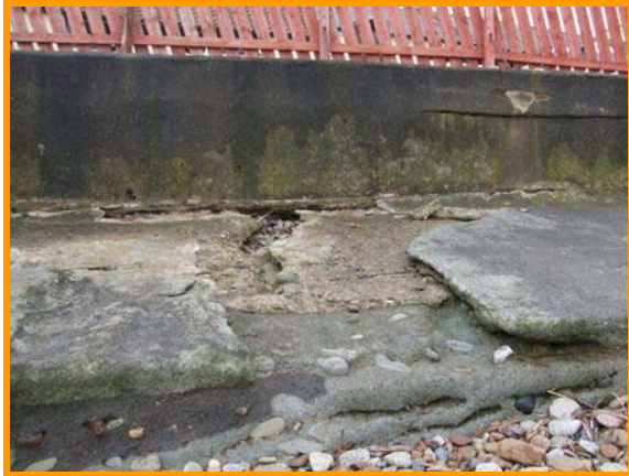
2008: Property at risk behind eroded concrete defences (Asset Ref No. 1221C901C0704C05)
