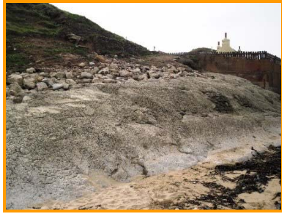
2010: Undercutting and excavation of concrete defences (Asset Ref No. 1221C901C0704C05)
