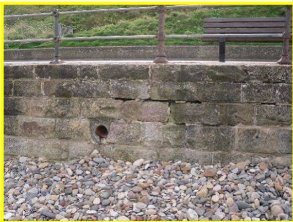
Example of area where repointing is needed (Asset Ref No 1221C901C0704C04)
