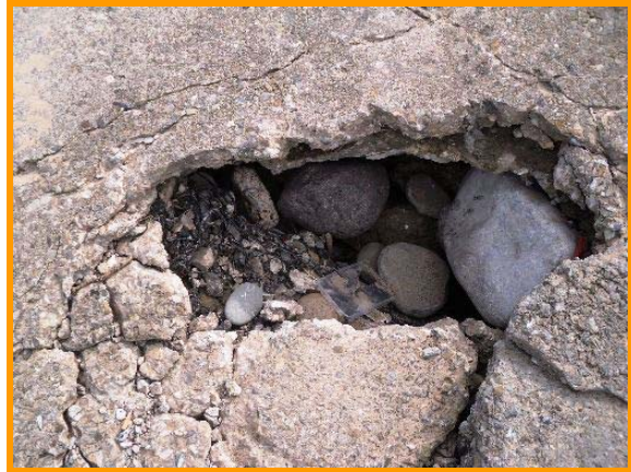
Void within slipway (Asset Ref No. 1221C901C0704C05)
