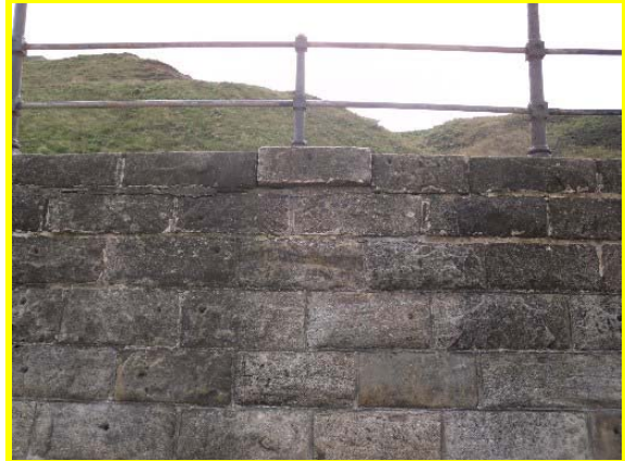
Example of area where coping is loose (Asset Ref No 1221C901C0704C04)
