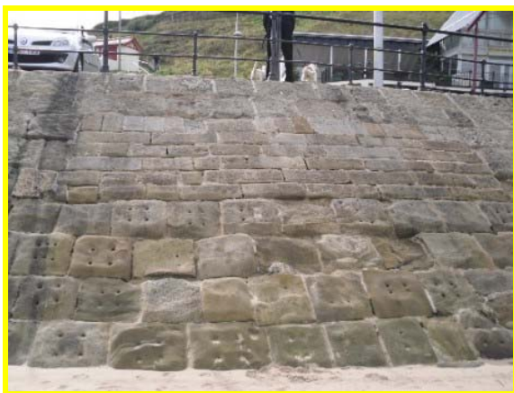
Area of repair, and potential area of deformation (Asset Ref No 1221C901C0704C01 )
