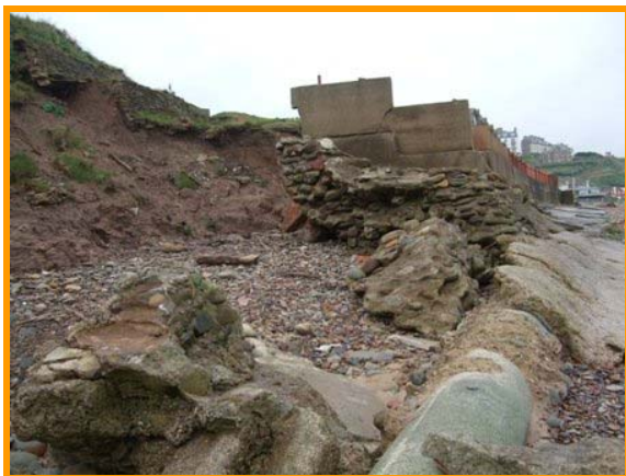
2008: Partial collapse of concrete defences and failure of unprotected cliffs above (Asset Ref No. 1221C901C0704C05)
