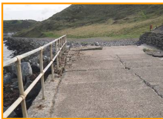
Landward end of jetty – showing movement (Asset Ref No. 1221D901D0201C02)
