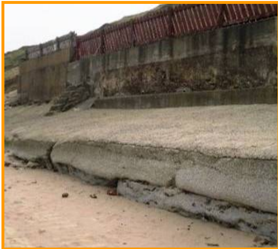
2010: Repairs visible, but defence still shows evidence of cracking and erosion (Asset Ref No. 1221C901C0704C05)
