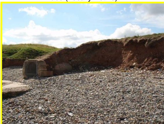
E52/10 Erosion of natural slopes surrounding outfall structure at Mill Howle (Locally Active)
