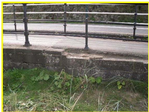
Example of area where coping is missing (Asset Ref No 1221C901C0704C06)
