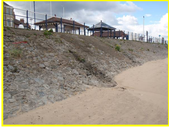
Loss of concrete render exposing grouted stone (Asset Ref No 12221C901C0601C01)
