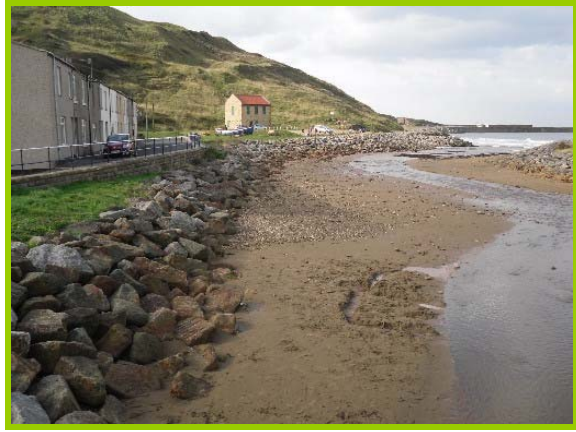
Rock armour along Beck with small wall behind in Skinningrove village (Asset Ref No. 1221D901D0202C02)
