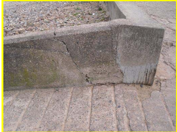
Cracked wing wall in slipway attached to sea wall at Hazel Grove Foot (Asset Ref No 1221C901C0703C02)
