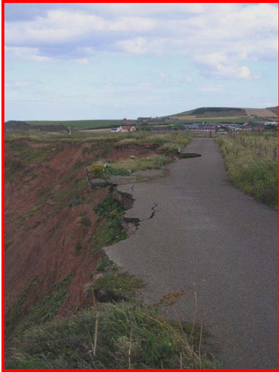
E59/3 ongoing loss of abandoned road at Cowbar (Totally Active)
