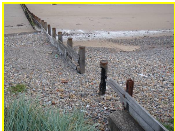
Fire damage and missing/broken timbers (Asset Ref No 1221C901C0701C01)
