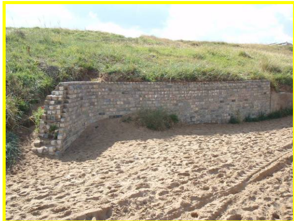
Masonry wall with cracks and missing masonry at seaward extent (Asset Ref No 12221C901C0702C01)
