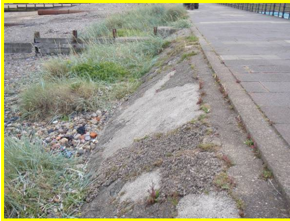
Missing concrete render – evidence of local patch repairs (Asset Ref No 1221C901C0701C01)
