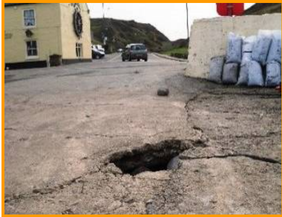
Void and cracking slipway (Asset Ref No. 1221C901C0704C05)
