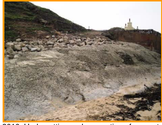
2010: Undercutting and excavation of concrete defences (Asset Ref No. 1221C901C0704C05)
