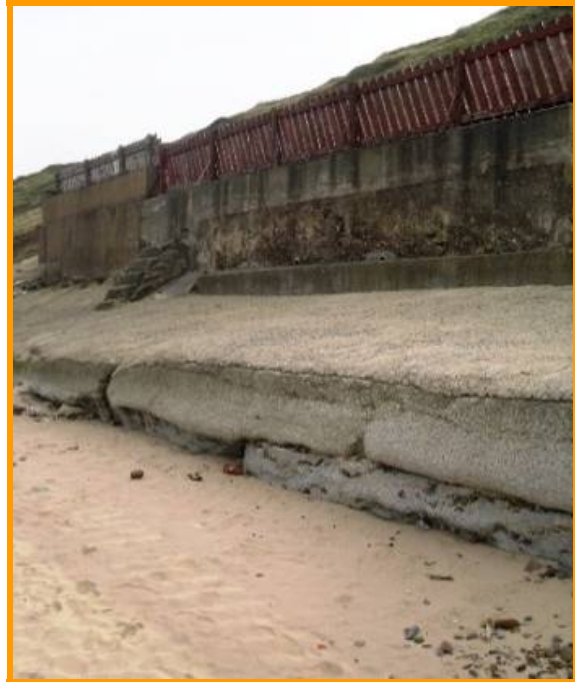
2010: Repairs visible, but defence still shows evidence of cracking and erosion (Asset Ref No. 1221C901C0704C05)
