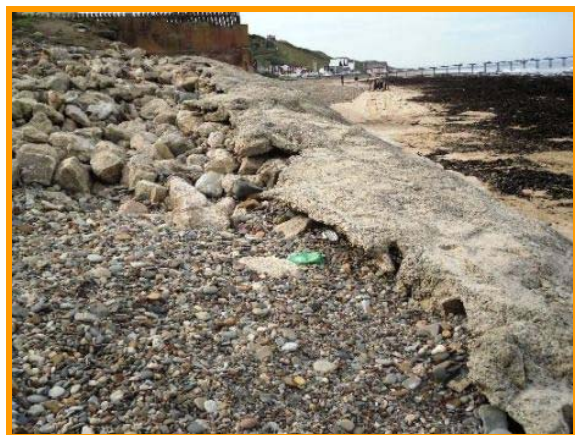
2010: Total collapse of part of concrete defences and failure of unprotected cliffs (Asset Ref No. 1221C901C0704C05)
