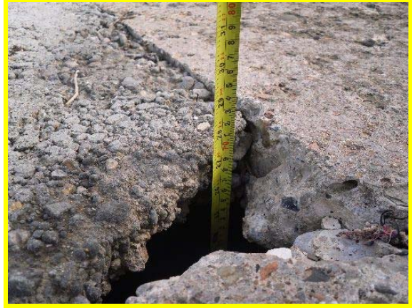
Void, showing 700mm depth (Asset Ref No. 1221D901D0202C03)
