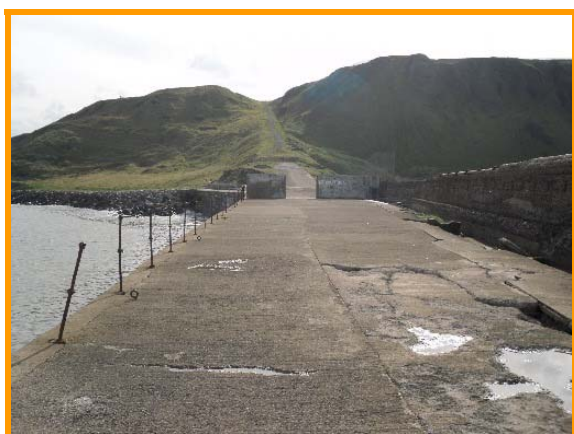
Looking landward along the jetty, showing open gates in background (Asset Ref No. 1221D901D0201C02)
