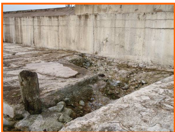
Voids present in deck - 2008 (Asset Ref No 12221C901C0506C01)
