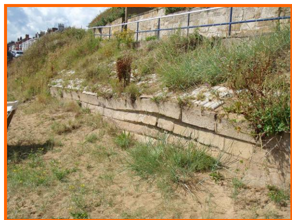
Local settlement of masonry structure (Asset Ref No 12221C901C0702C02)
