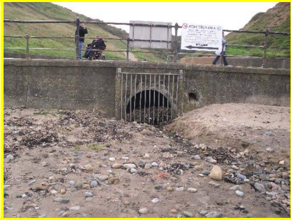
Partially blinded outfall exiting through sea wall at Hazel Grove Foot (Asset Ref No 1221C901C0703C02)
