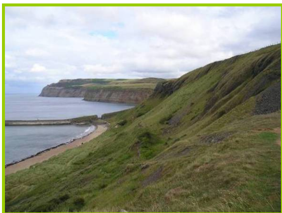
E56/2a looking southeast towards Skinningrove, showing shallow vegetated slopes and dunes at the toe (Inactive)
