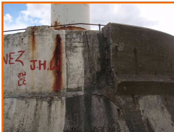
Missing pre-cast concrete units at head of breakwater (Asset Ref No 12221C901C0506C01)
