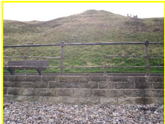
One section where a section of hand rail is missing (Asset Ref No 1221C901C0704C04)
